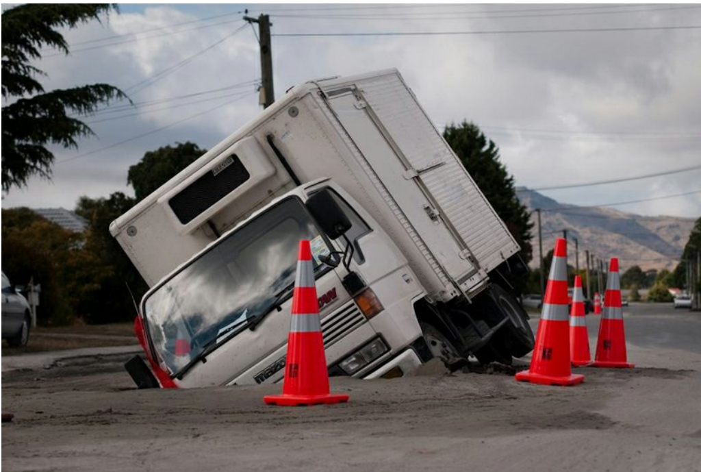
Figure 1. Road slumping after 2010 earthquake. 1
